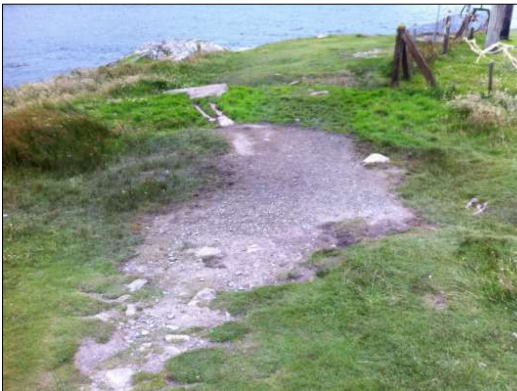
Figure 3.48 Erosion of grass cover and exposure of underlying soil at Garnish
