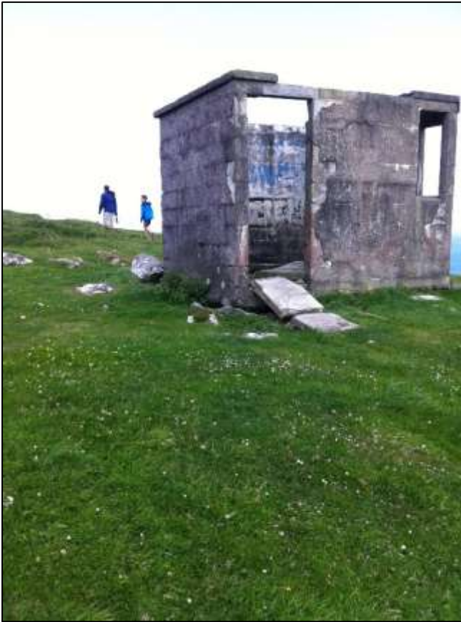
Figure 3.21 Observation building at Brandon point, the roof has collapsed in and the structure is in poor condition
