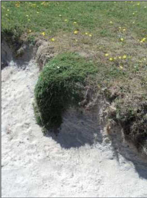
Figure 3.40 Erosion at edges of walkway, may have been happening prior to installation of walkway at Barley Cove
