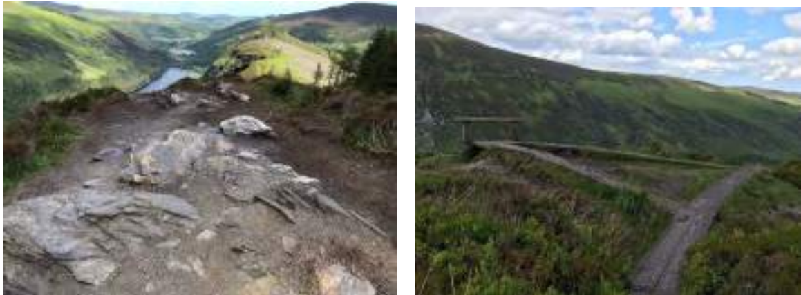
Fig. 22 Areas shown signs of erosion due to walkers stepping off the trail to take photos.
