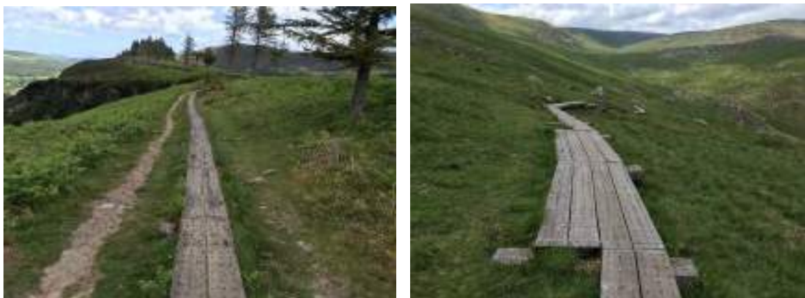
Fig. 21 Damaged surface running parallel to the boardwalk where it's not wide enough for walkers to pass. Where the boardwalk has been widened this is having a positive impact.
