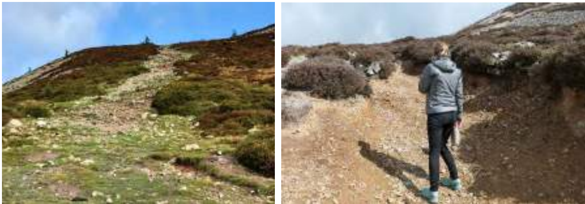
Fig. 4 Vegetation stripped away to leave a rough stony path and large gully to the right of the path created and vulnerable to natural erosion processes.
