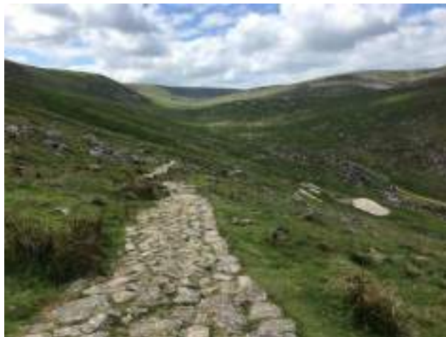
Fig. 19: Previously eroded trail that has been stone paved just after where the boardwalk stops
