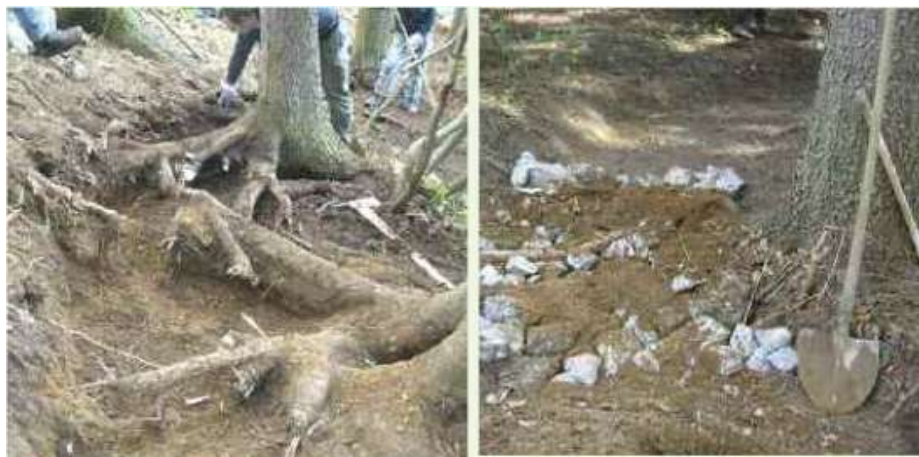
Figure 7 Excavation of anchor roots by hand and packing of anchor roots by hand
