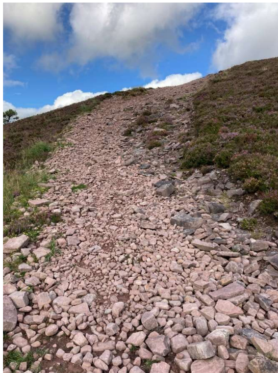
Figure 27 Existing section of BBW identified as requiring stone pitching
