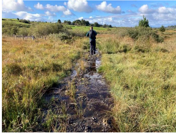
Figure 16 Existing gravel trail with no geotextile resulting in trail sinkage
